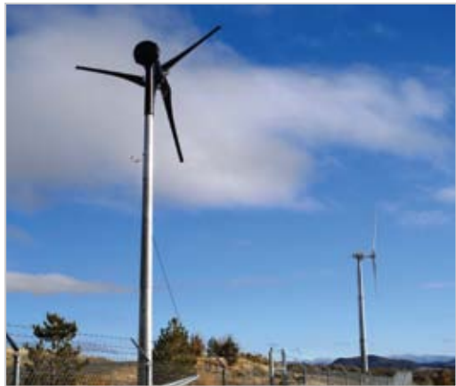
Ameresco installed two wind turbines at the City of Reno Stead Waste Water Treatment Plant.
