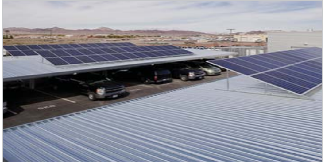
North Community Police Substation upgraded its solar energy system with the help of ARRA funds. The city's electric bill will be about $5,000 cheaper.
